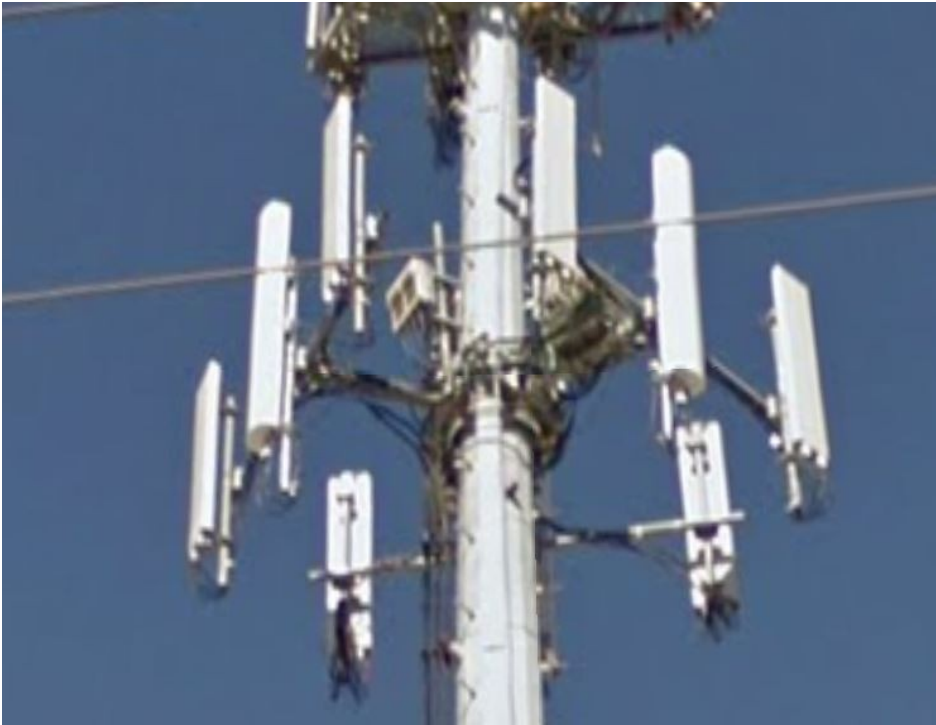
Figure 3. Note the box enclosure with vents in the center of this image. This is an AT&T equipment tower, owned by Crown Castle.
